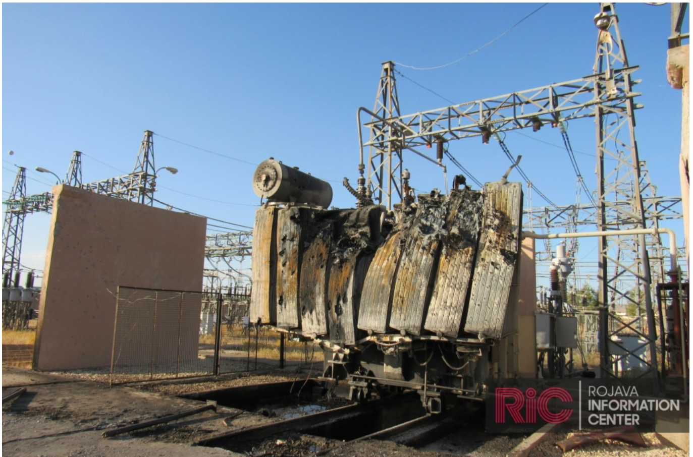
Electricity station, Qamishlo
