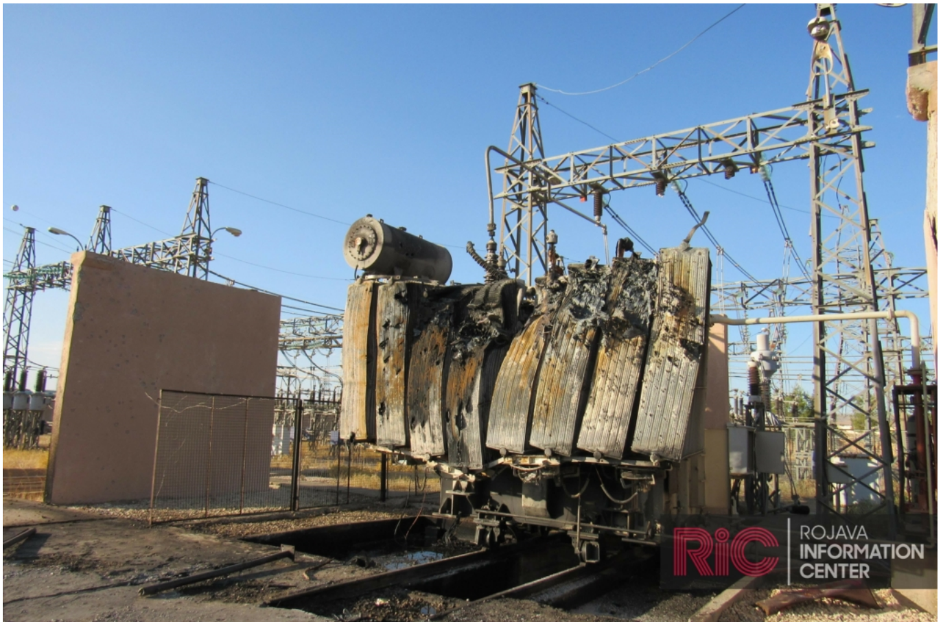
Electricity station, Qamishlo
