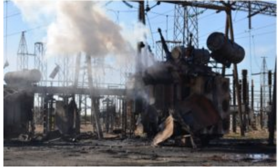
Damage caused by Turkish air attacks on civilian electricity infrastructure in Suwaydiyah North & East Syria. Photo: Rojava Information Center
