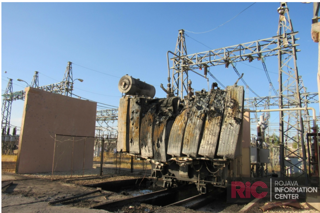
Electricity station, Qamishlo
